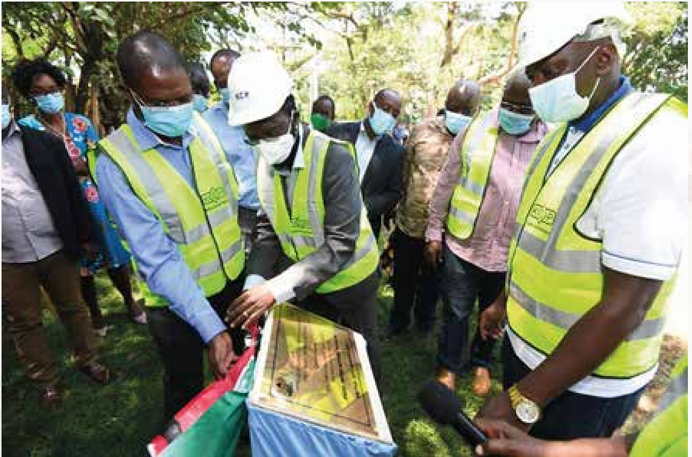
Kisumu Governor Prof. Anyang' Nyong'o and Speaker Hon Elisha Oraro unveil the plaque to commemorate the groundbreaking of construction of the speaker's official residence.
