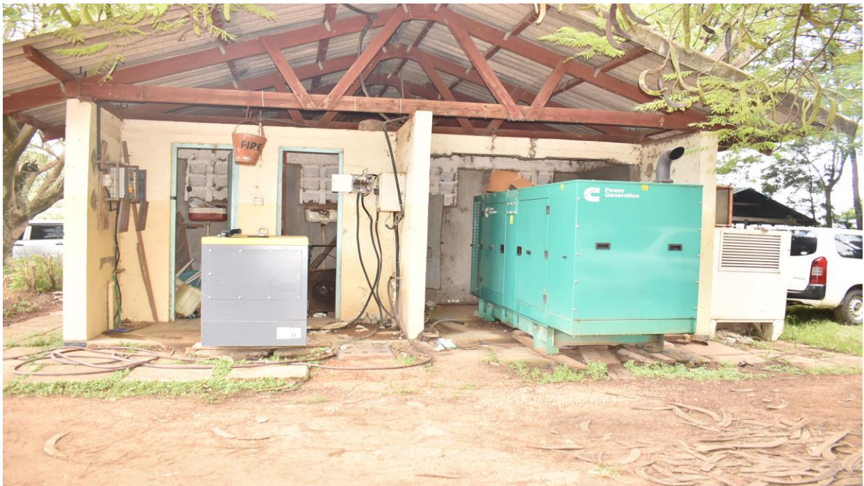
The three generators at the facility.
