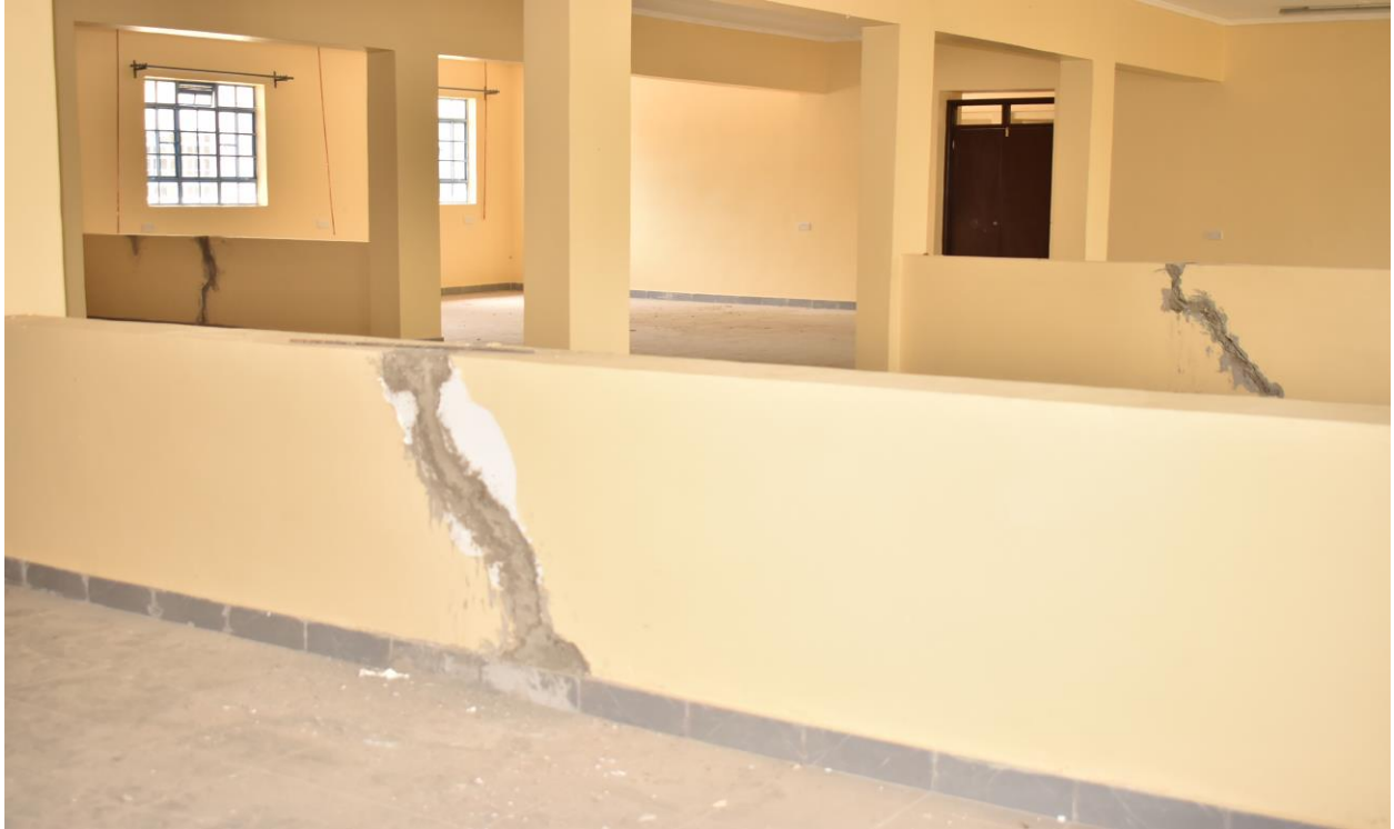
More cracks on the interior of the maternity complex.
