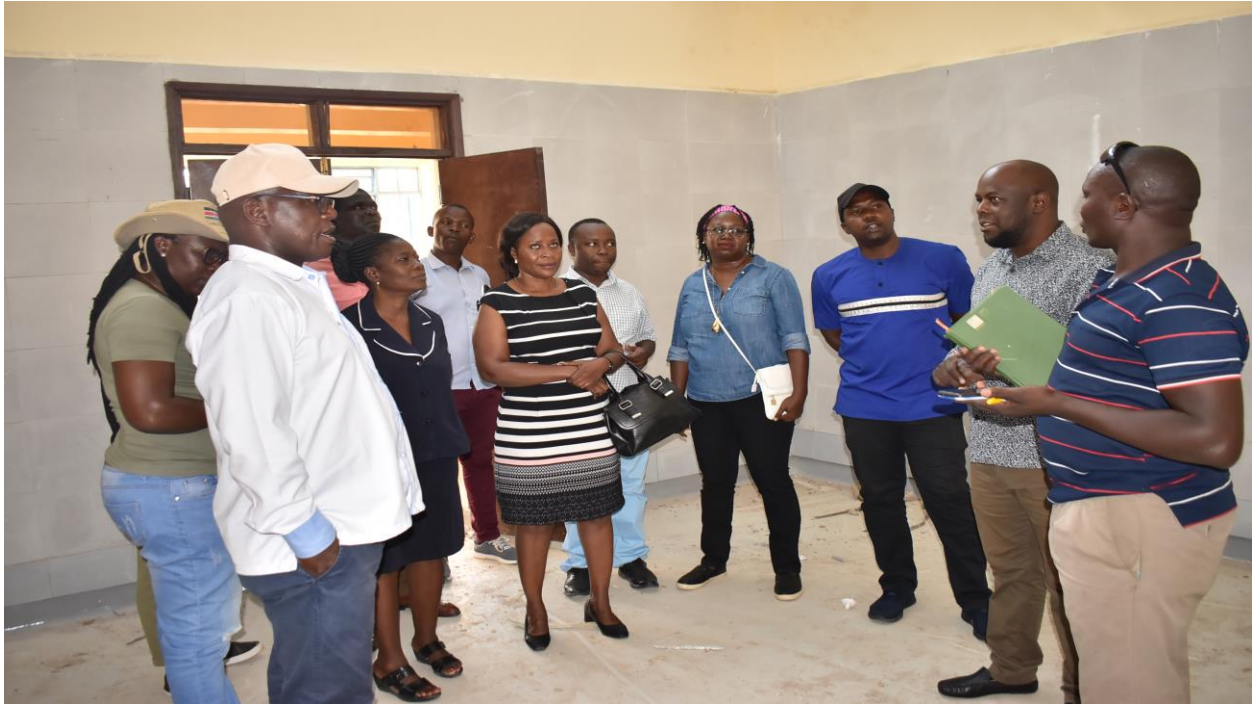
The Contractor's site manager (in striped t-shirt), the medical superintendent and Committee members inside the maternity complex under construction
