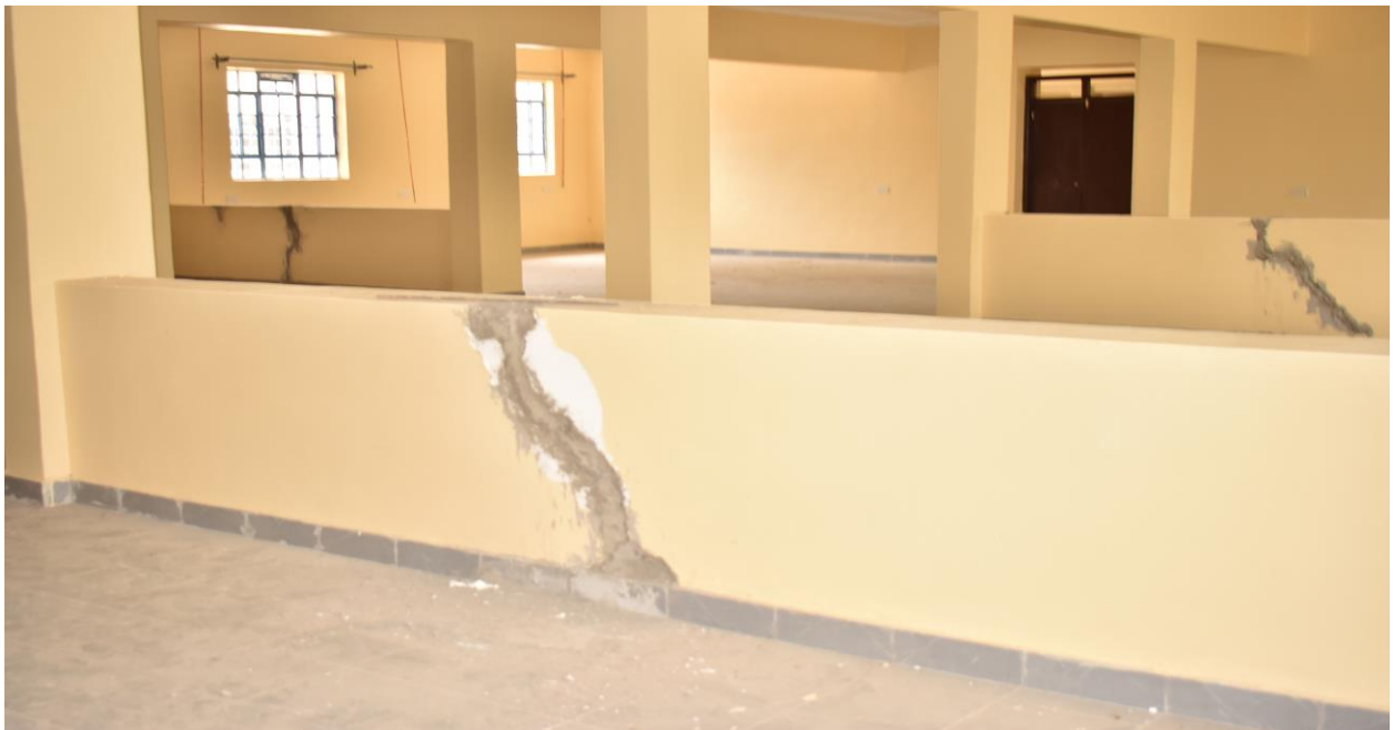
More cracks on the interior of the maternity complex.
