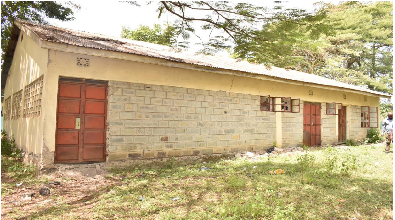
Another condemned building.
