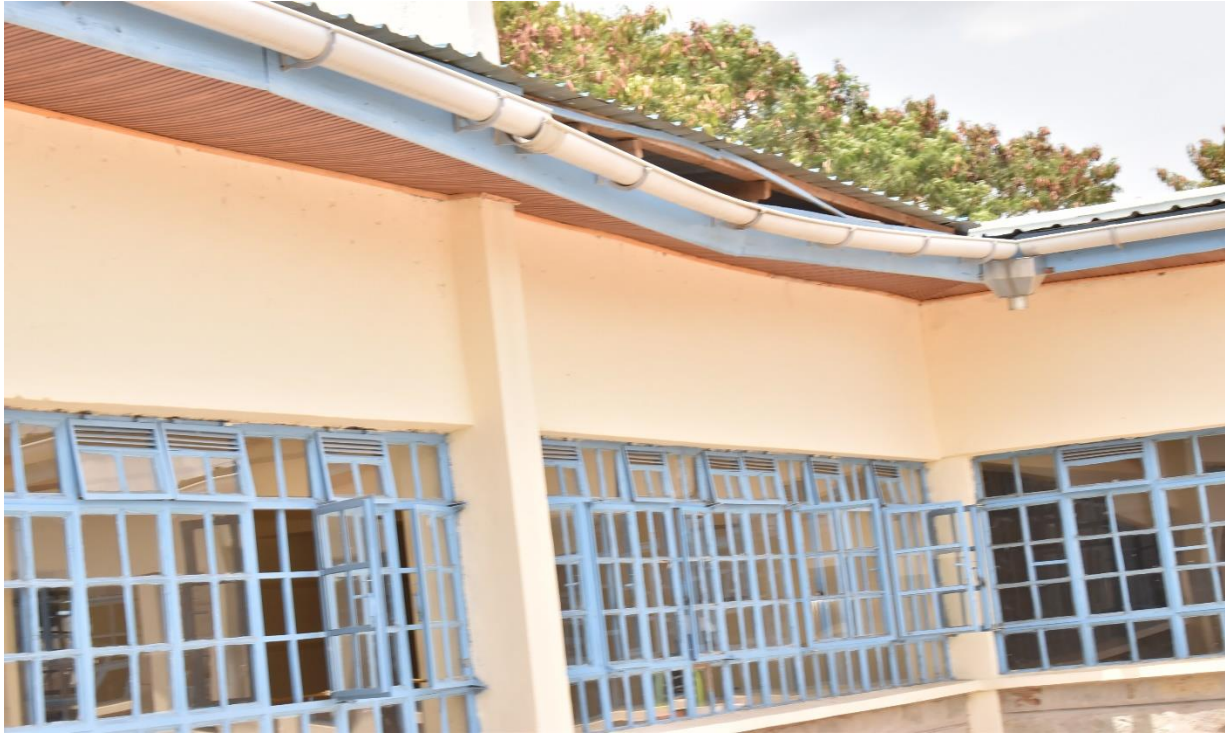
Gutter falling off - Maternity complex under construction.
