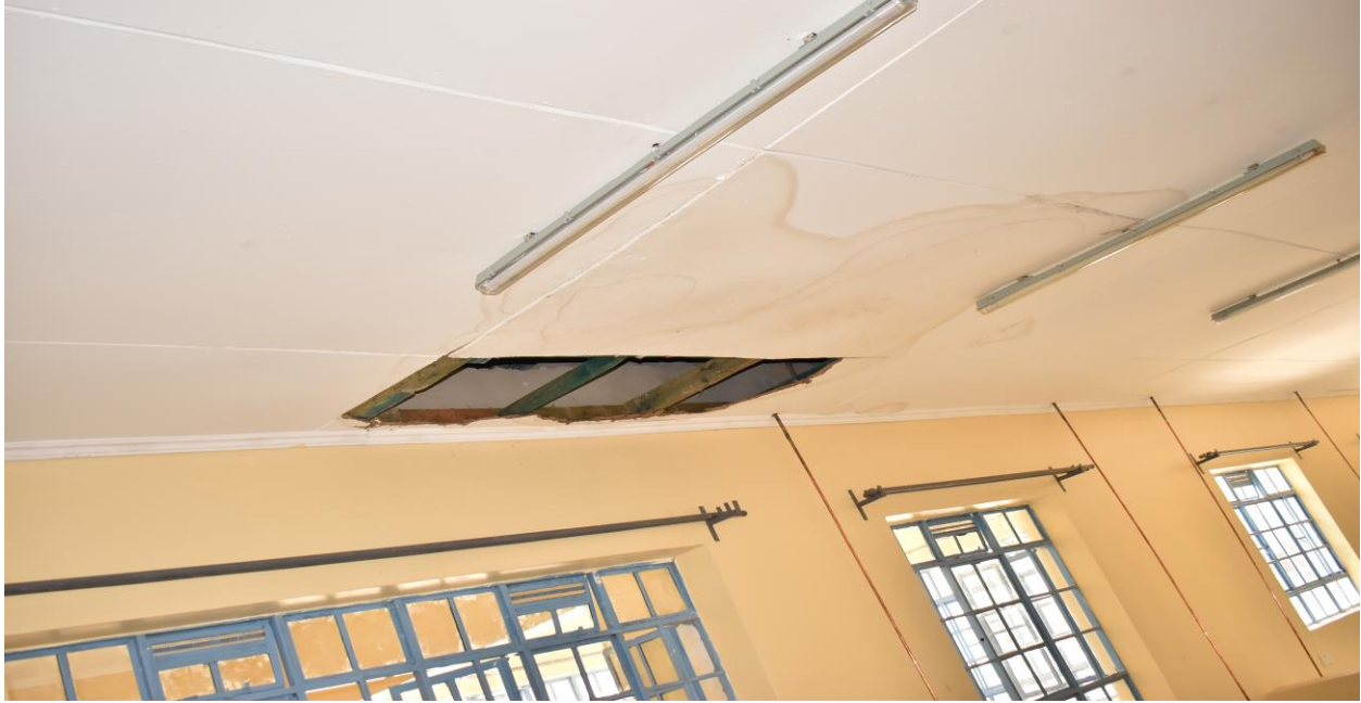
Discoloured ceiling board as a result of leaking roof.
