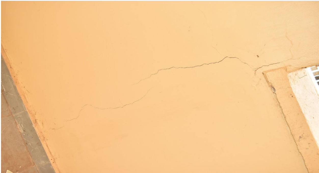
Cracked wall – interior of the maternity complex under construction.
